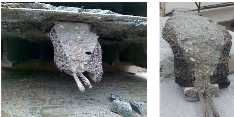
Fig. 3.38. View of shear failure of the PC girder in slab element [30]
