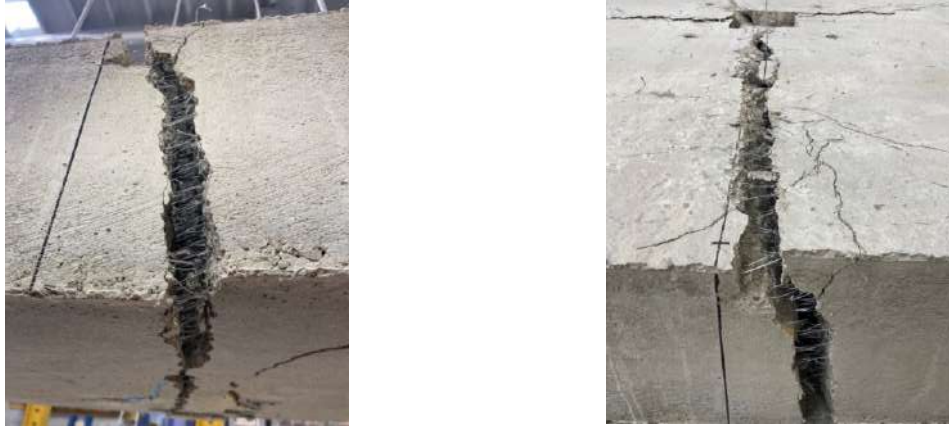
Fig. 5.25 Synthetic fibers PM maintaining the structural integrity of the tested slab 2.2
