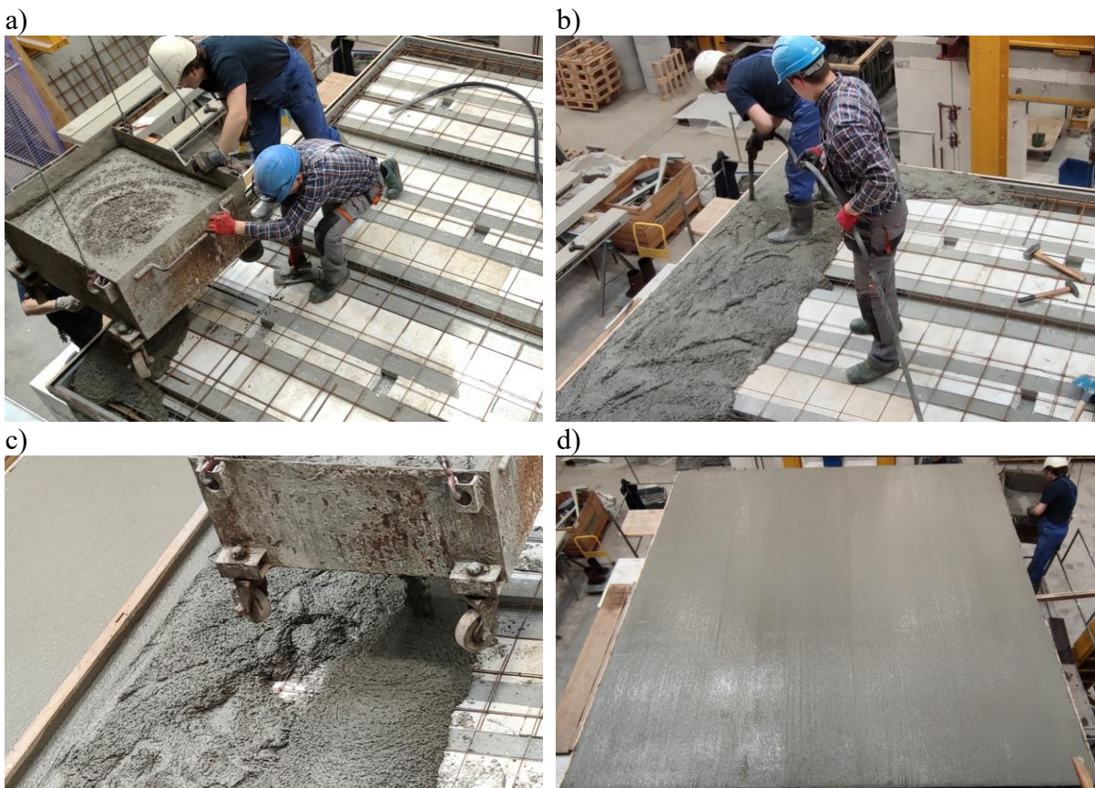
Fig. 4.12 Concreting the slab and the upper beam: a) concrete bucket, b) compaction of concrete using a vibrator, c) laying the concrete mix, d) finishing of concrete
