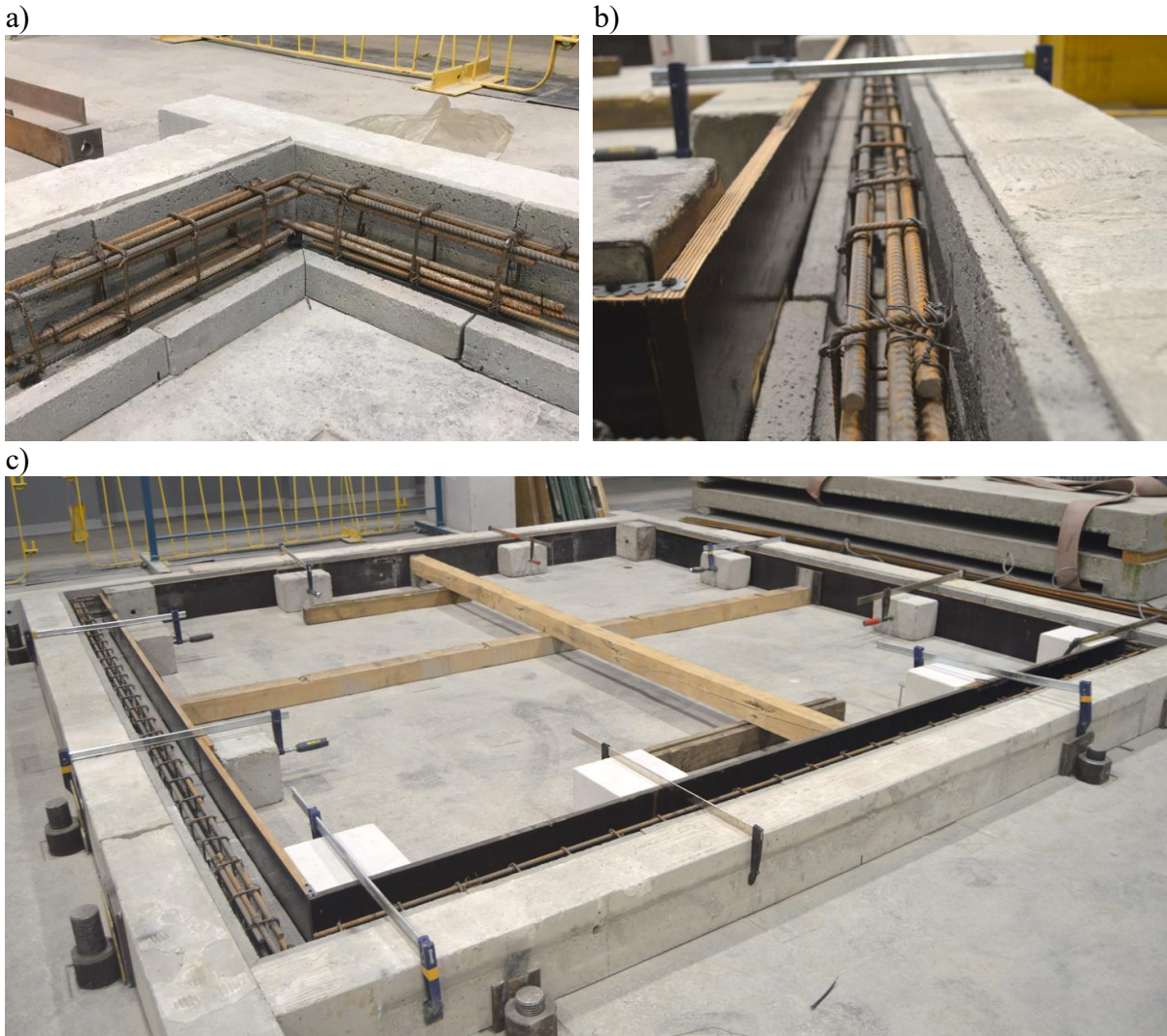
Fig. 4.2 Execution of construction details of the bottom beam: a) corner reinforcement, b) main bars with stirrups, c) bottom beam formwork
