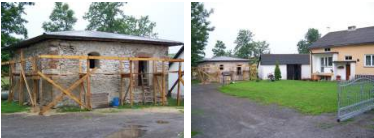
Fig. 162. Remainings of the castle in Kwaśniów Dolny under conservation works in 2010, source: https://zamki.rotmanka.com/ , [access: 12.07.2021]
