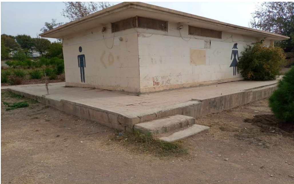
Figure 4. An example of stairs on the main path to the restrooms in Azadi Park, Iraq.
