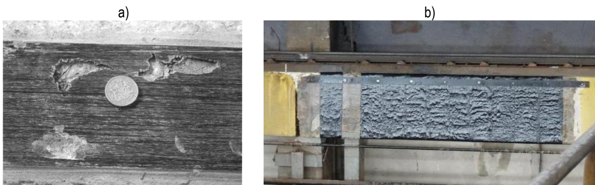
Fig. 2.18 a) Examples of defects in CFRP strip [N18] b) poorly bonded CFRP mat [courtesy of Kakuza M.]
