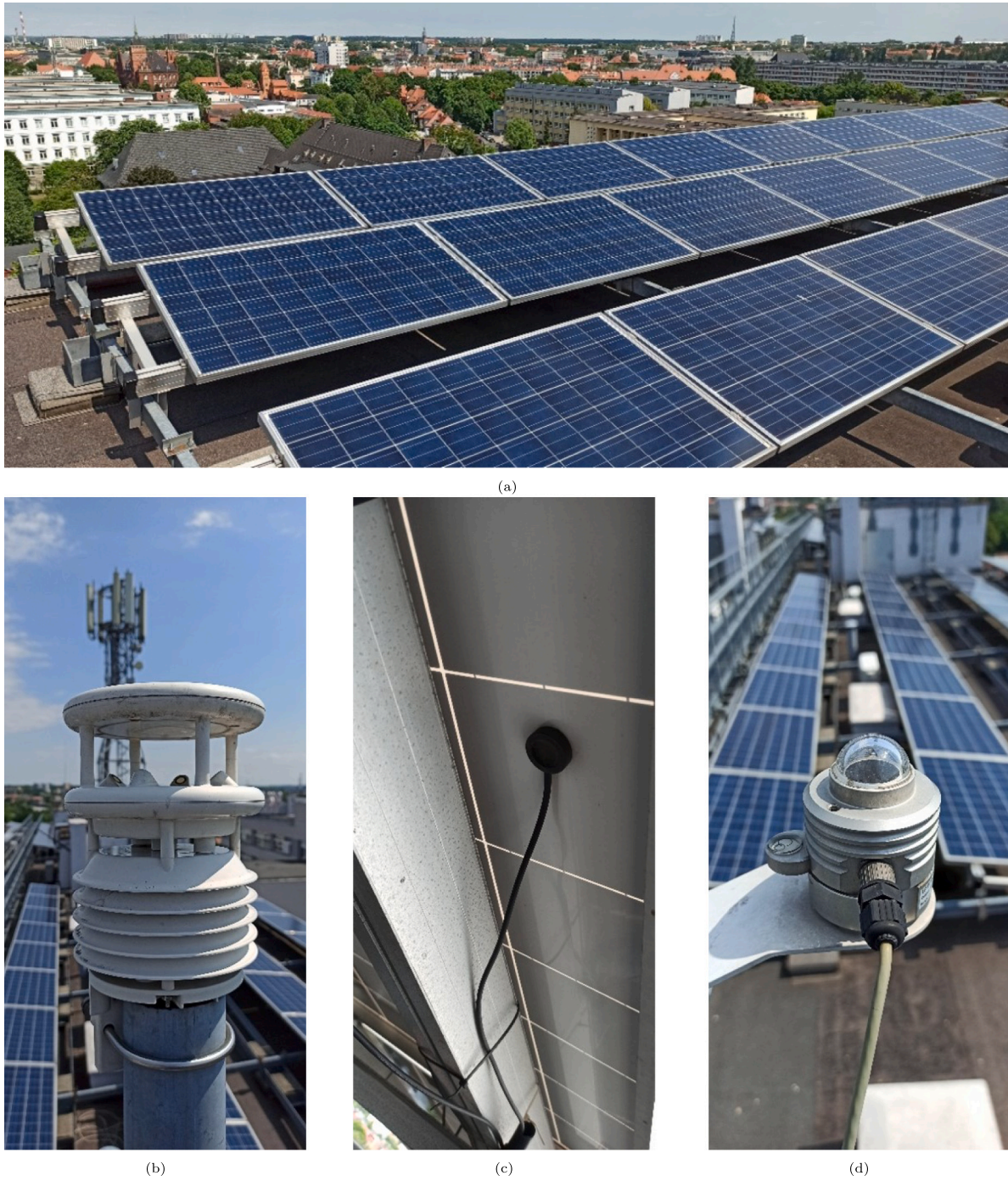
Fig. 1. The PV installation (a), weather station (b), external temperature sensor for PV temperature measurement (c), and pyranometer (d) on the roof of the building of the Faculty of Automatic Control, Electronics, and Computer Science of the Silesian University of Technology in Gliwice, Poland.
